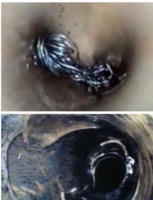
Figure 5. Casing collapse of a 9-5/8” production casing in a high-temperature geothermal well with remains of slick line from a stuck logging tool. The collapse was punched out leaving the anchor casing exposed to the wellbore fluids, by courtesy of Reykjavik Energy and ON Power.
